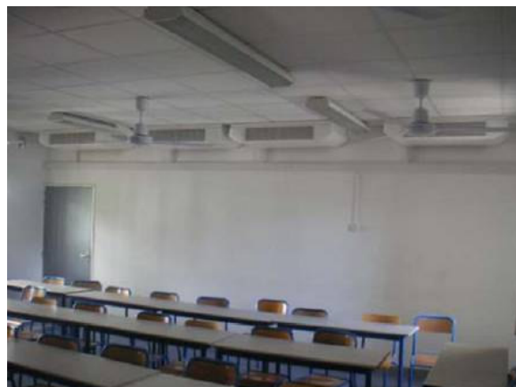
Figure 3.32 - Example of an Solar-Assisted Air-conditioning application in La Réunion, France (small island near Africa) [25]. This project was executed by Schüco International KG. At this picture the fan-coil units in the Auditorium (ca. 200 m²) are visible.
