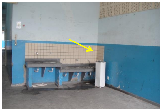
Photo 6- Adapted installation of the drinking water fountain in the recreation area of school A. Source: By the researcher, 2017.
