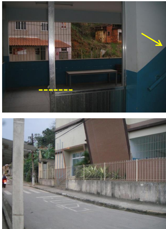
Photos 3 and 4- The height of the door's glass is too low, same height as the handrail. Main entrance of school B, with glass door. Source: By the researcher, 2017.
